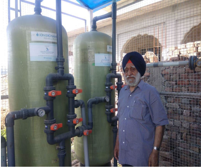
Prof. Virk visiting Ion Exchange Plant at Kuralian village (Ajnala block of Amritsar district)
